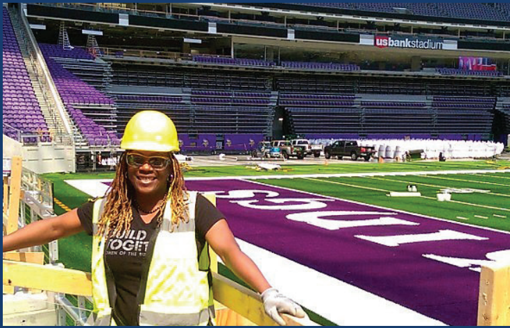
LeWanda Harper, Laborers Local 563 journey member, at work at the new Vikings stadium
